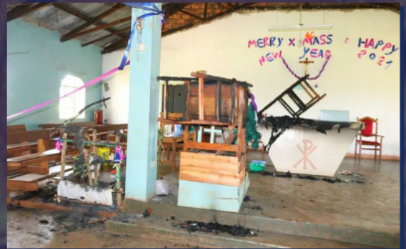
A church in Kenya after fire
