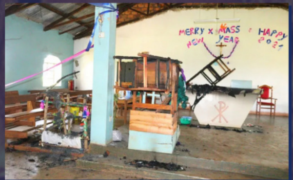
A church in Kenya after fire
